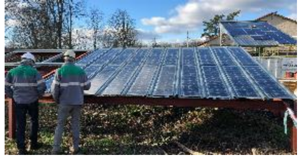
FIGURE 2 : (FOREGROUND) PVSTEEL MS GEN0.2 MODULES, WITH (BACKGROUND) CRYSTALLINE MODULES
